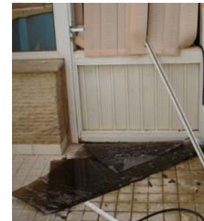
Blast Damage – Tech
